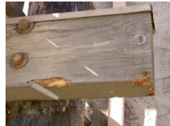
Photo: 26 - Drywood termite damage, Incisitermes , family Kalotermitidae Photo: Dr. Vernard R. Lewis
